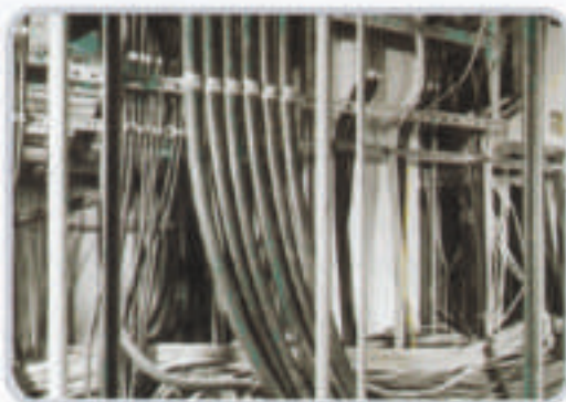
电缆布线复杂,火灾荷载高 Cable layout is complex,high fire load
